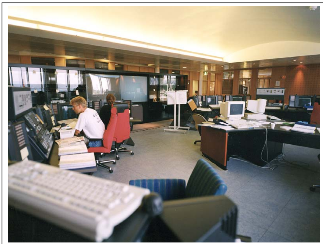
Control Room – Photo: Øyvind Hagen, Statoil
